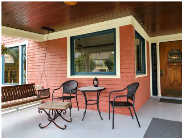
STAINED CEILING + ENTRY DOORS
