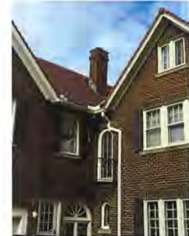
ALL NEW BORAL TRIM TO BE PAINTED TO MATCH EXISTING HOUSE TRIM COLOR
