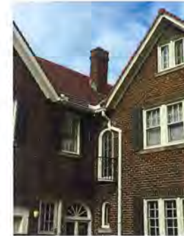
ALL NEW BORAL TRIM TO BE PAINTED TO MATCH EXISTING HOUSE TRIM COLOR
