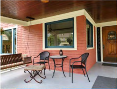
STAINED CEILING + ENTRY DOORS
