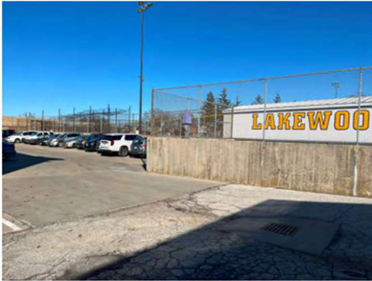
Looking east at the retaining wall and elevated ball field east of the project site
