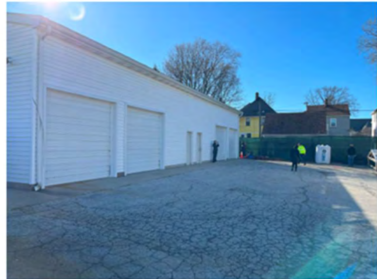
Looking west at the existing storage building to be demolished, south of the D Building
