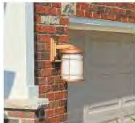
EXISTING LIGHT FIXTURE
