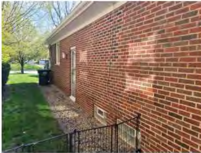
EXISTING CONDITIONS - SIDE OF HOUSE
