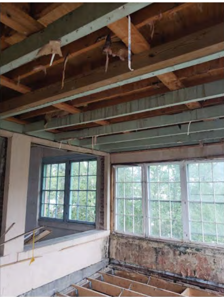
Lakewood's building inspector visited the site and agreed that the area above the garage seems to have once been open with a pergola (see green painted framing)
