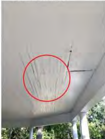
Current Porch Damage:
