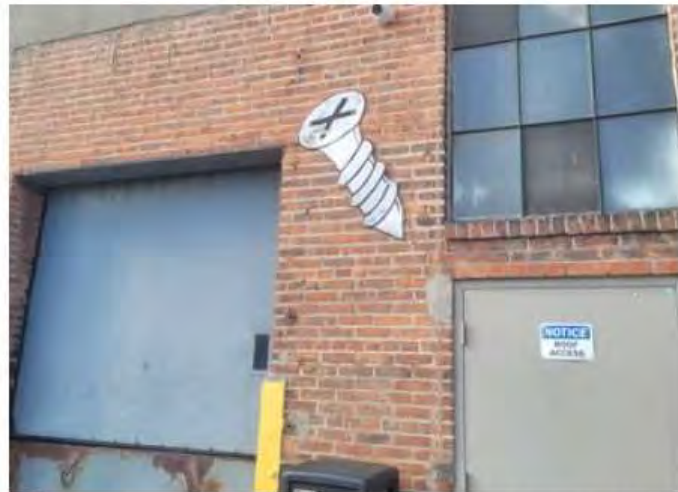
14 Remove existing screw graphic above East Stairwell door. patch/ repair masonry as required.
