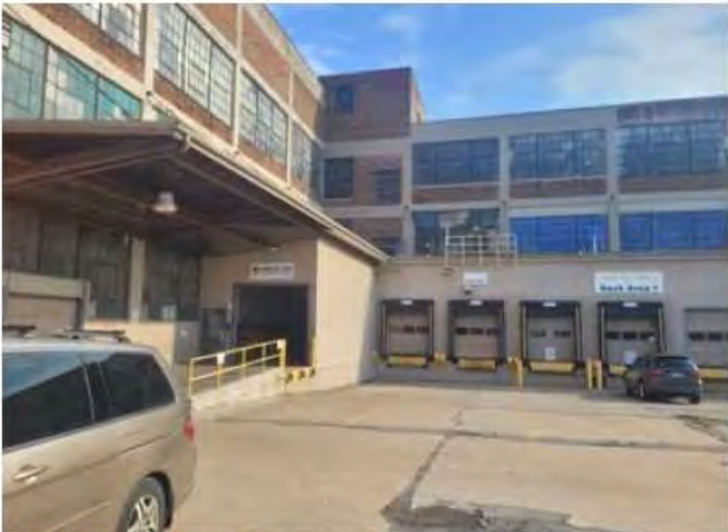
4 5 6 Remove existing Choctaw-Kaul, Tenant Dock, and Dock Area 1 signage. Patch/ repair masonry as required.
