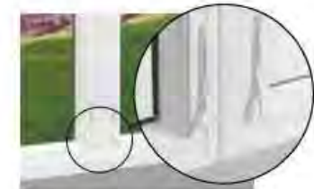
Appearance of a non-reinforced joint
