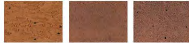
IRON SPOT FLASHED FLASHED WITH IRON SPOT
