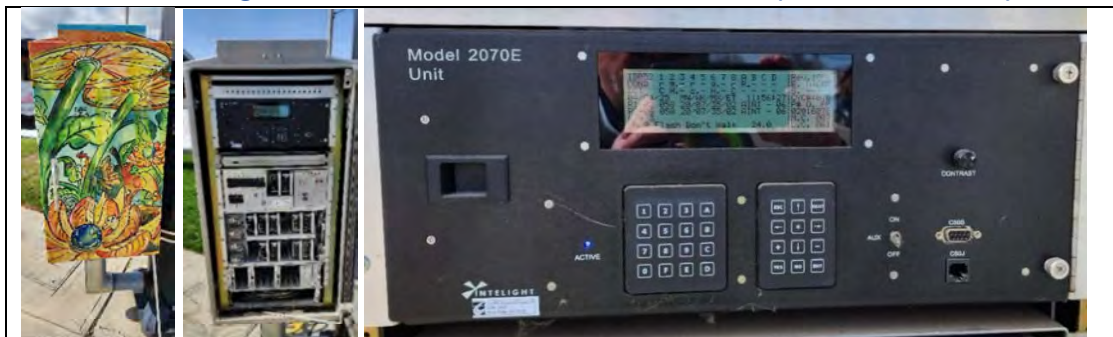
Figure 8 – Madison Ave & Hilliard Rd/Carabel Ave (2070 controller Unit)
