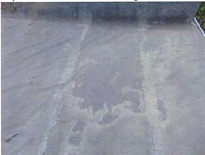
The roll roofing on the Eastern most section of the flat roof is beyond its useful lifespan and should be replaced to prevent moisture from entering the structure.
