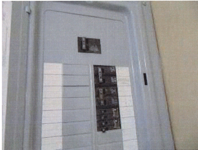
Main disconnect is located in the main distribution panel
