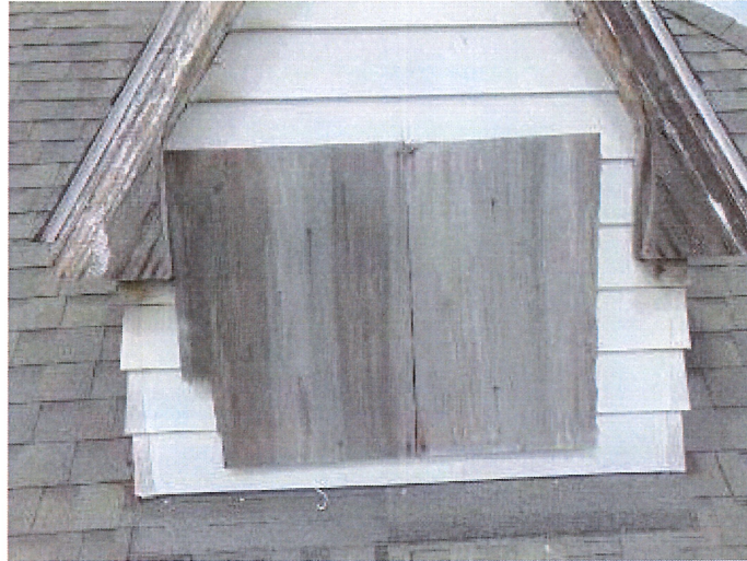
A window on the upper East side was boarded up.
