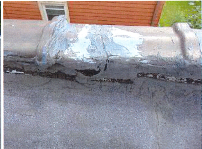
The roll roofing on the Eastern most section of the flat roof is beyond its useful lifespan and should be replaced to prevent moisture from entering the structure.
