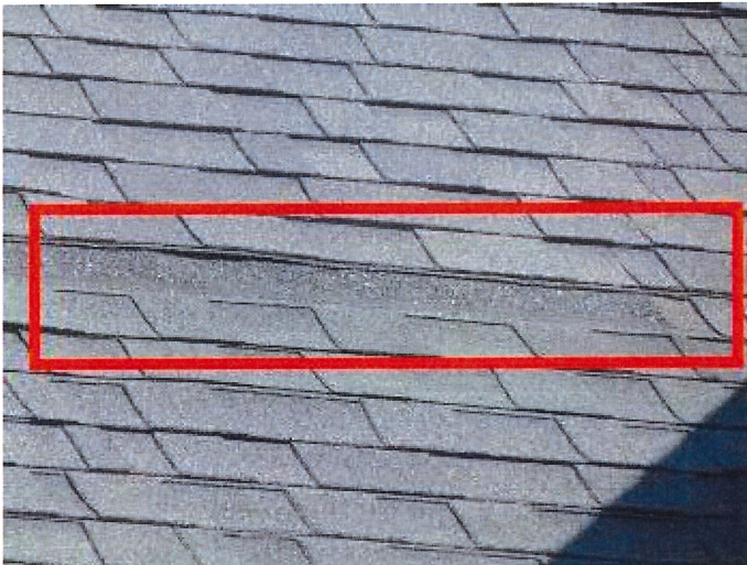
Missing asphalt shingles were noted on the South side of the main section of the roof. I recommend having new shingles installed in these areas to prevent moisture from entering the structure.
