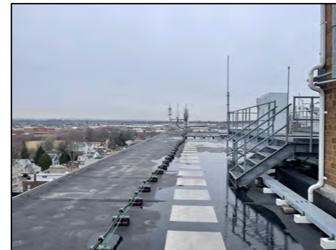
Existing Cable Run (Other Carrier)
