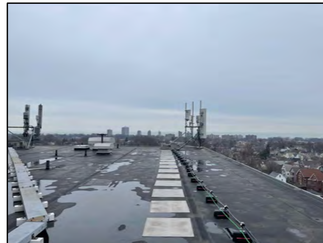
Existing Cable Run (Other Carrier)
