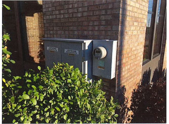
Electrical meter along west side of building
