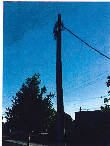
Power pole along Parkhaven Row
