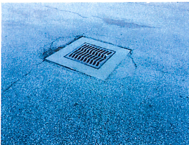
Catch basin in parking lot
