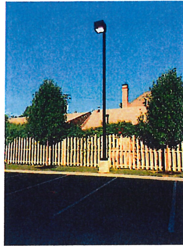
Parking lot light pole
