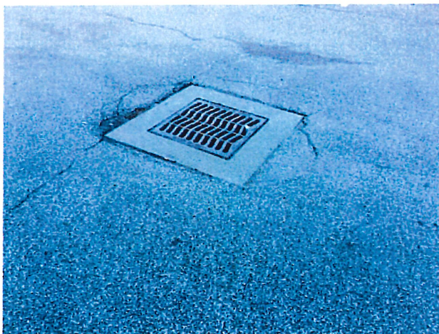
Catch basin in parking lot
