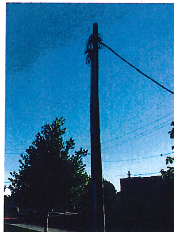
Power pole along Parkhaven Row
