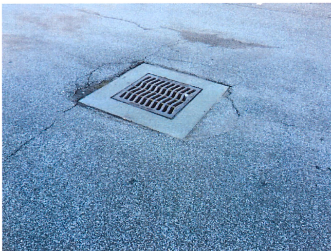
Catch basin in parking lot
