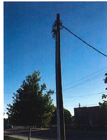
Power pole along Parkhaven Row
