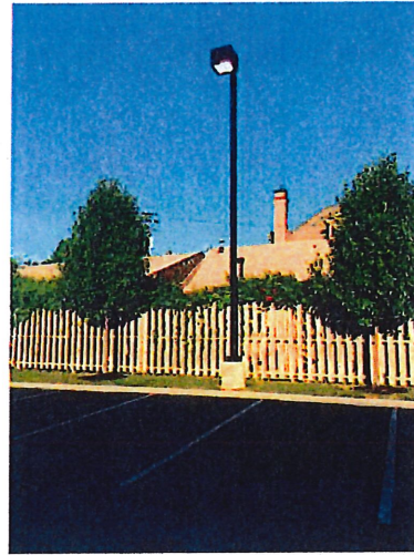
Parking lot light pole
