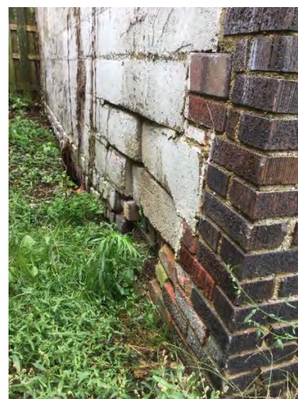
Garage north wall damage
