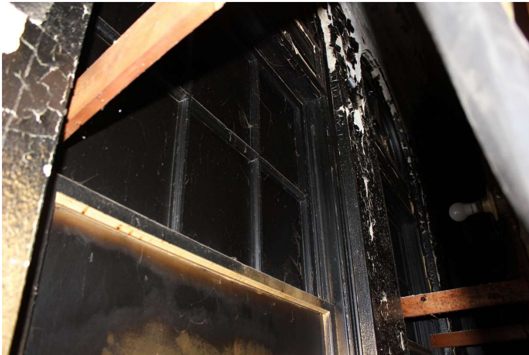
Photo 10: Original windows hidden behind added wall (c.d. NE)
