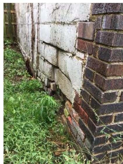
Garage north wall damage
