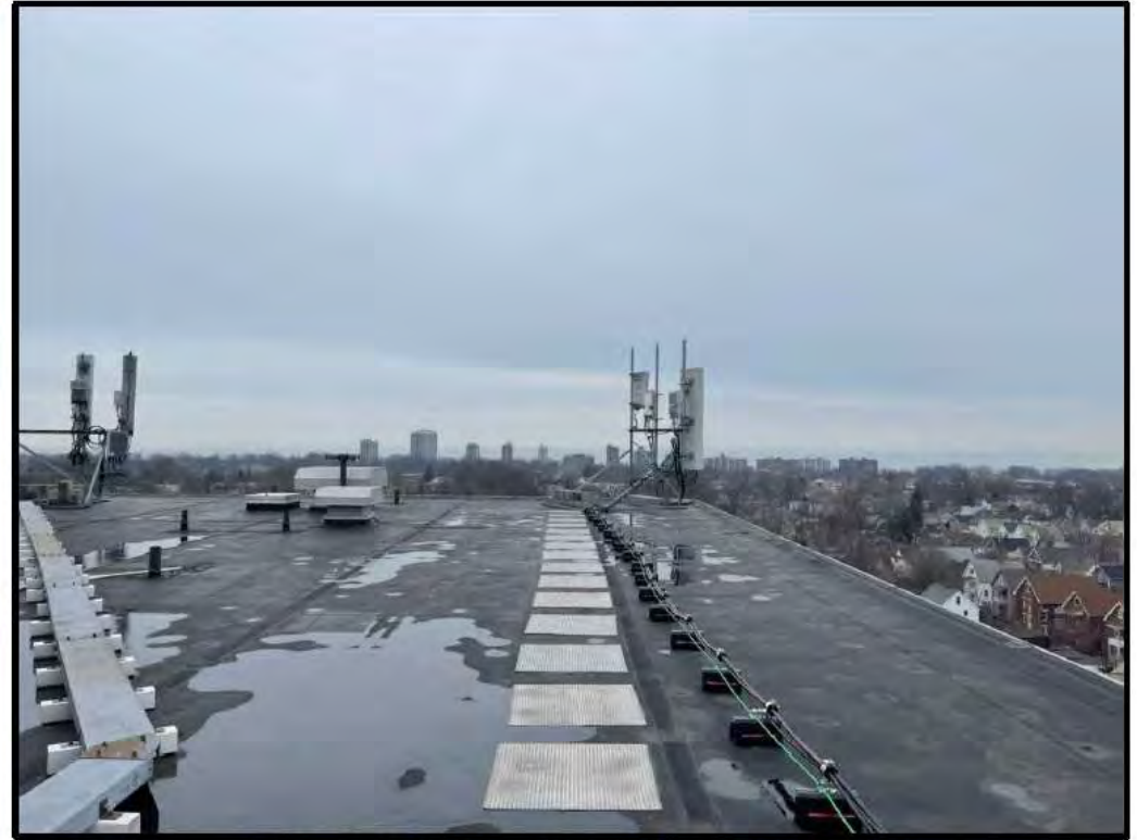
Existing Cable Run (Other Carrier)
