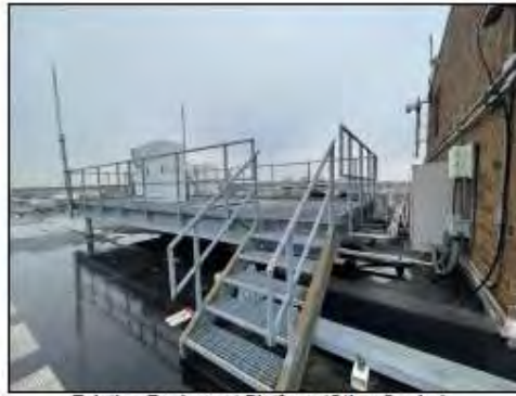
Existing Equipment Platform (Other Carrier)
