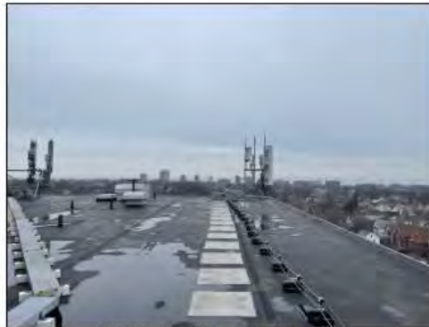
Existing Cable Run (Other Carrier)
