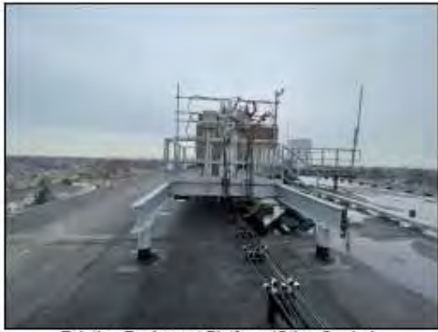
Existing Equipment Platform (Other Carrier)
