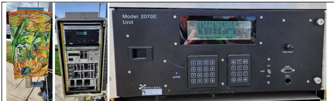
Figure 8 – Madison Ave & Hilliard Rd/Carabel Ave (2070 controller Unit)
