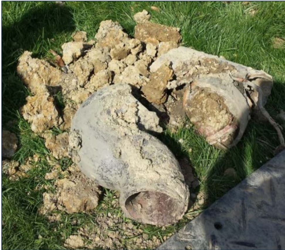
Figure 5-2 Trap Clogged With Sediment
