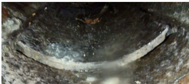
Post Televising Invert Plate Conditions
