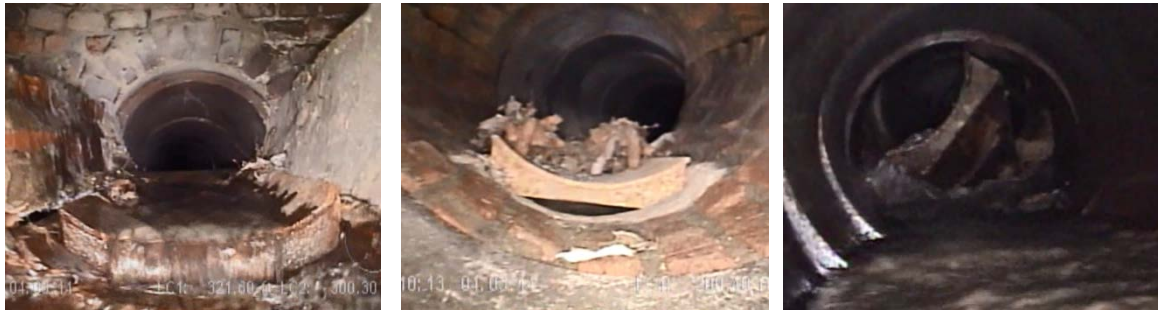
Figure 2-3 Invert Plate Conditions
