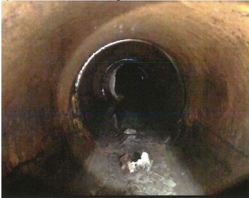
3) Storm inlet debris looking south:
