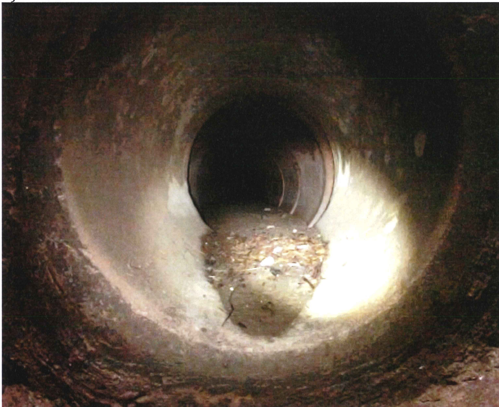
6) Western Inlet – 1"-2" of debris:
