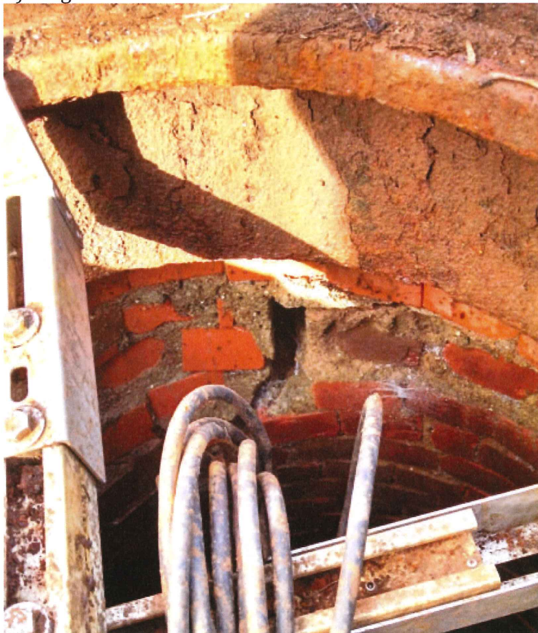
4) Large crack in brick cone near rim:
